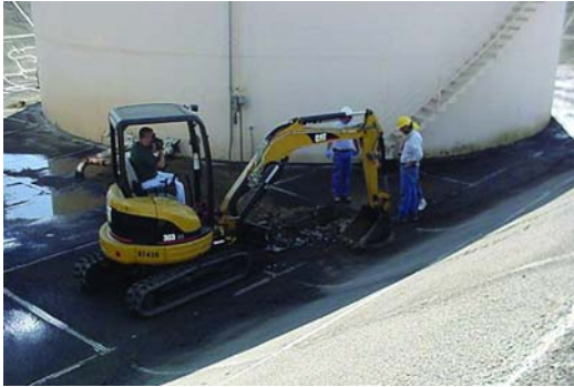
Above ground storage tank in Spokane.
